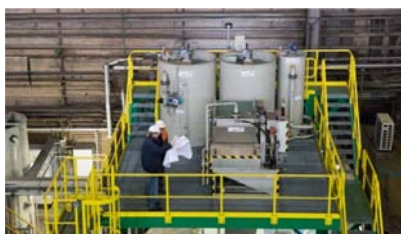
Chemical-physical treatment plant removes chromium-3 and formic acid from the wastewater
