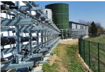
Photo: Wastewater from fruit processing is reliably purified to ensure that it meets the required limit values.
