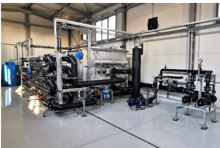
Photo: A Flomar flotation plant sits at the heart of the wastewater treatment solution.
