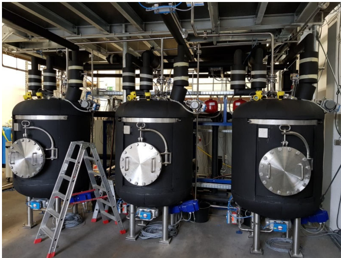
Image: During the installation of the SteriFix wastewater disinfection plant at RIVM in Utrecht.
