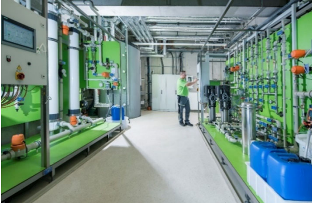
Image: Central EnviroFALK water treatment plant according to DIN EN ISO 15883 for the isolation ward in a hospital.
