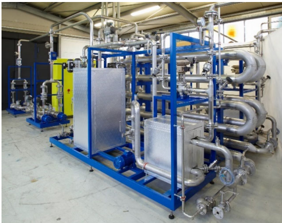
Image: EnviroDTS SteriFix E15000 wastewater sterilisation plant for safe inactivation of active components in wastewater.
