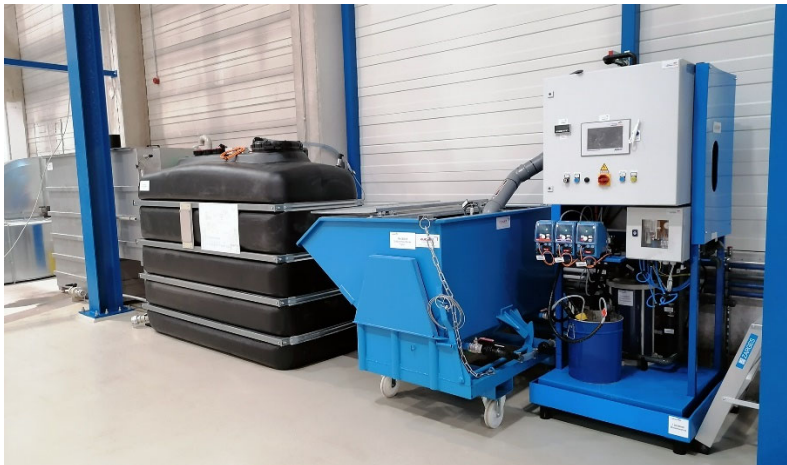
Image: Lugan plant with sludge tipping container, retention tank and high performance separator for treating wastewater from the workshops' cleaning processes.
