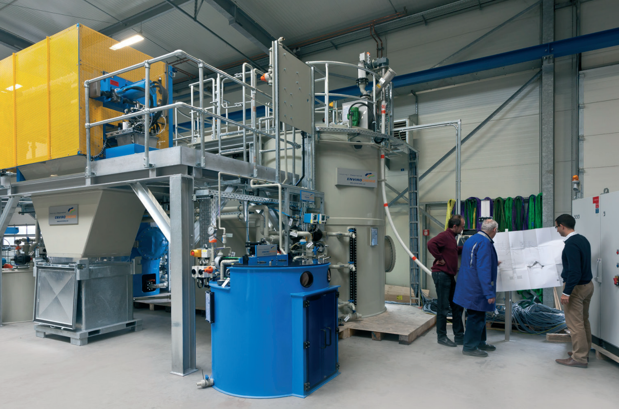
Envochem® chemical physical wastewater treatment plant ready for FAT
